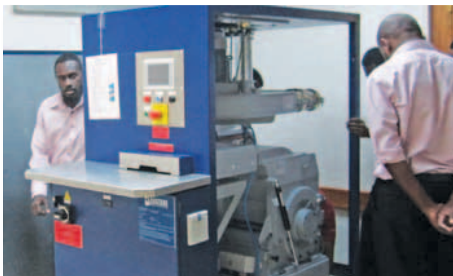
Installing the Bank's note shredding machine
